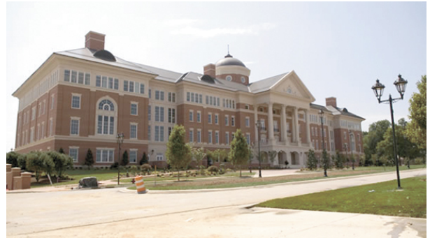
Construction slowdown: The NCRC will offer more than a million square feet of lab and office space when complete
